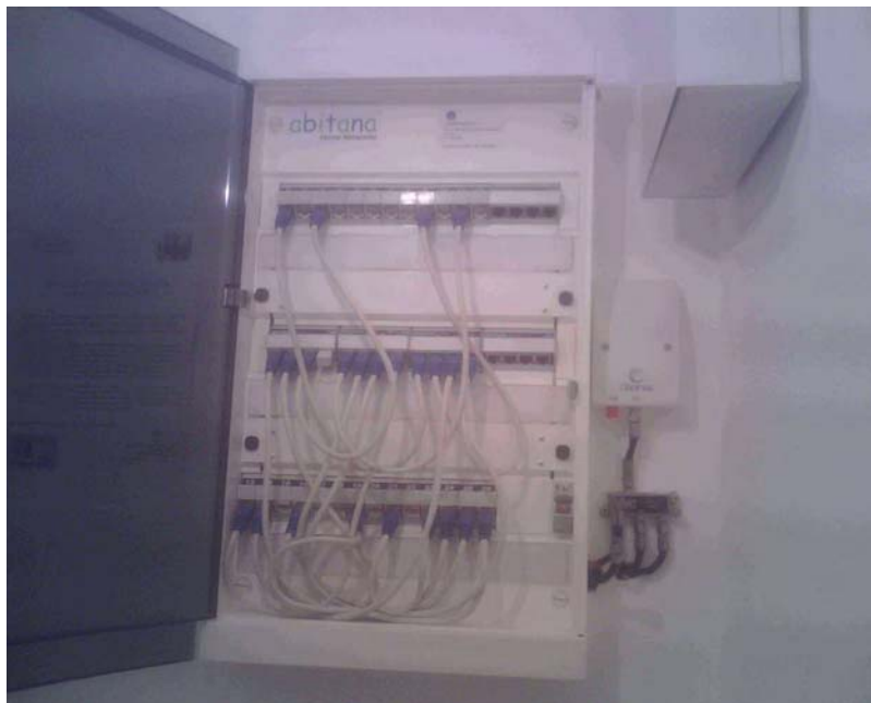
Figure 15 . Example of a Communications Panel
